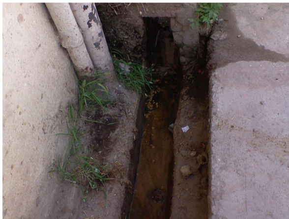
Excreta Coming out in open drain from ILCS Unit
